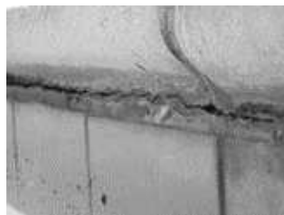
Tile at coping.
