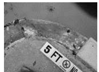
Coping broken off.
