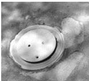
Pop-outs near drain.
